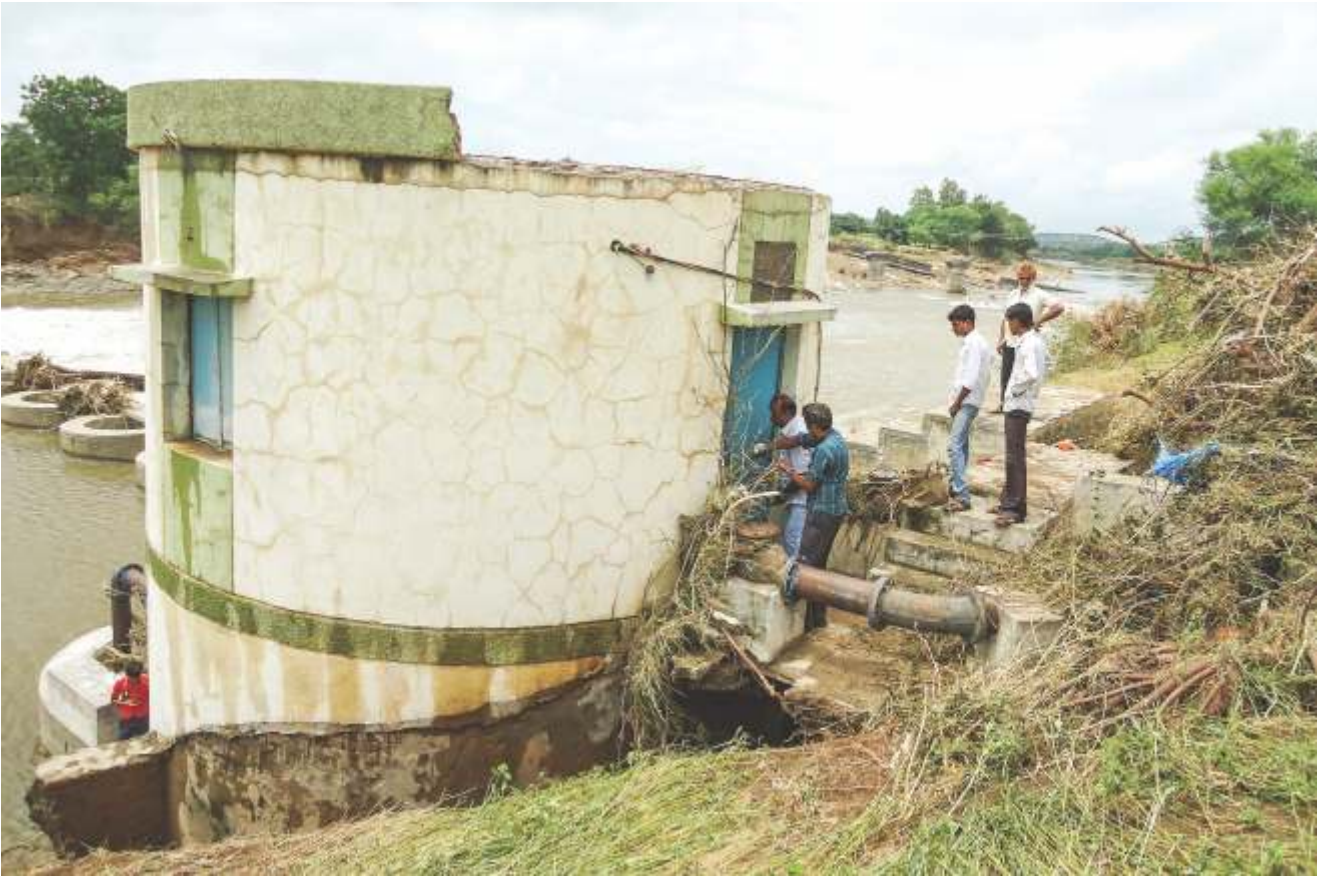
Flood damaged pumping station and delivery pipe of Vanjharia Lift Irrigation Scheme, Dahod
