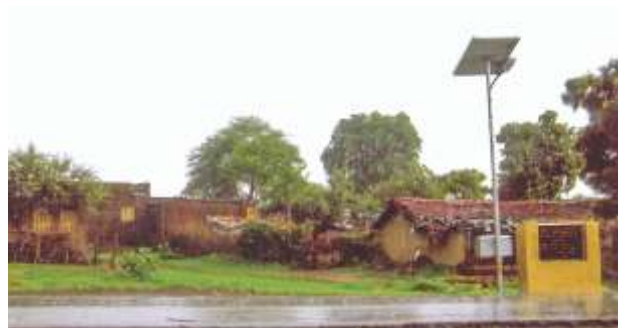
Solar street light installed at village Gordhanpura, Sitamau district Mandsaur, Madhya Pradesh under Integrated Watershed Development Project
